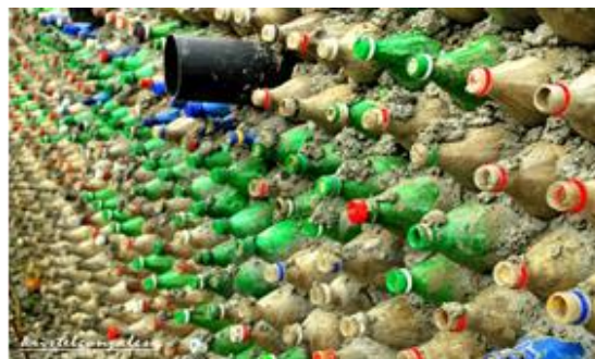
Figure 1 Inhabitat, Asia's First School Made of Plastic Bottle is 3X Stronger than Concrete, by Yuka Yuneda
