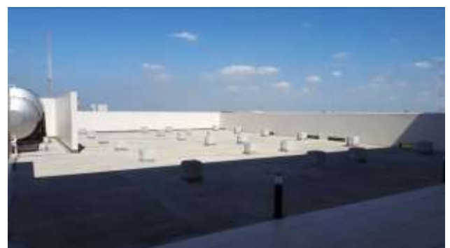
Figure 8. View of a portion of the roof deck area of the UPCA Studio Laboratory Building showing the pedestals for solar panels and water storage tanks.
