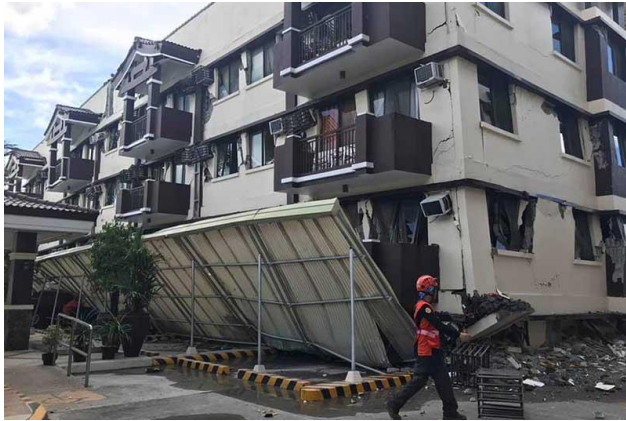
Figure 8. Damage from several earthquakes that hit the study area shortly before the survey was conducted.
