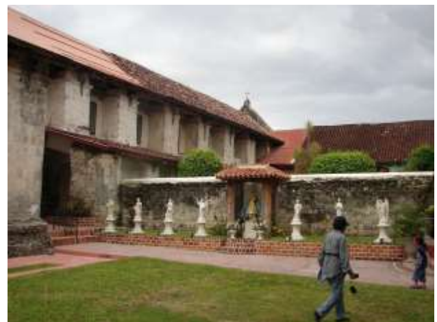
Figure 1. Boljoon church, erroneous roofing.
