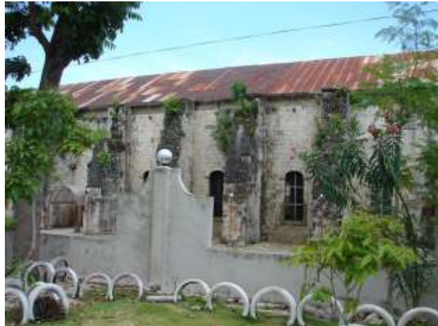
Figure 2. Samboan Church showing the lack of maintenance.
