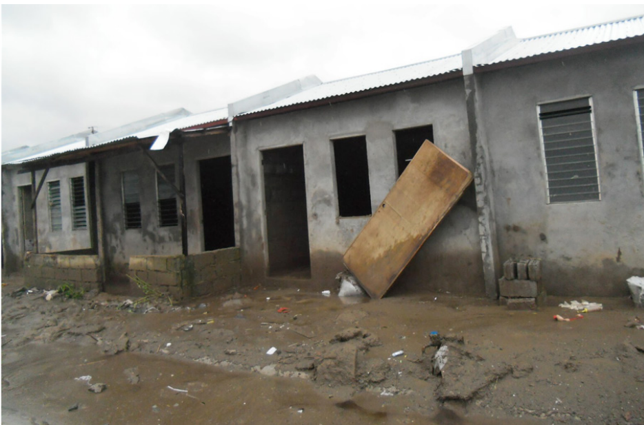
Figure 4. Housing units in Phase 1K2 after the 2012 monsoon rains. Photo from SIKKAD-K3.
